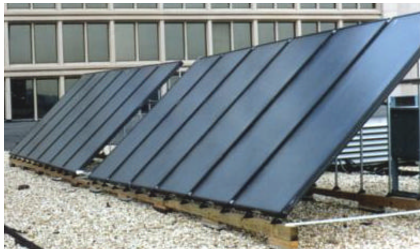
Fig.13.3: Solar water heater used in a) homes; and b) commercial establishments
