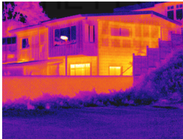
Fig.12.2: An IR scan of a house shows missing insulation above one window (dark blue)
