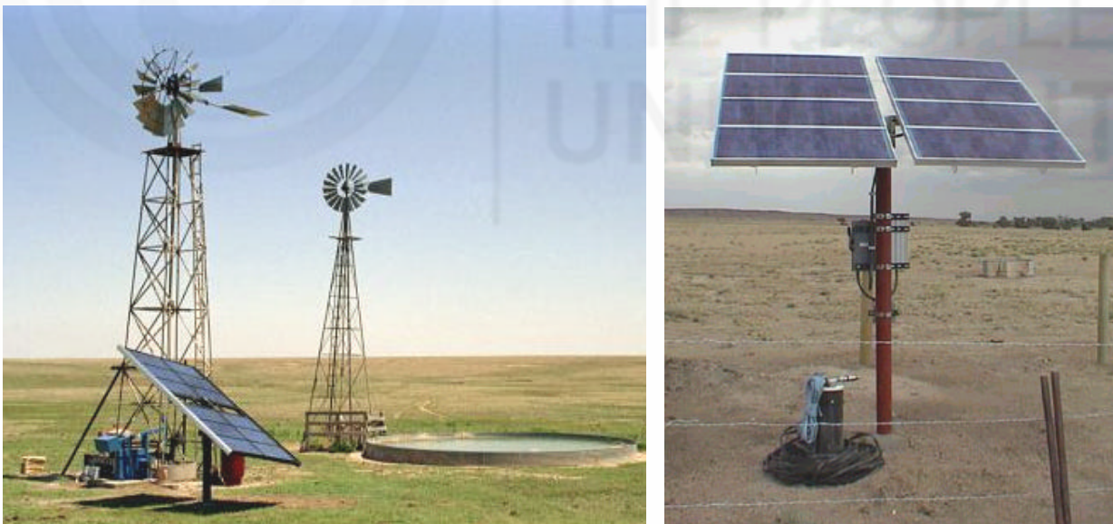
Fig.9.11: Solar water pumps
